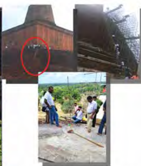
Fig.2: Crack appeared on the Stupa and the team visiting the location.
