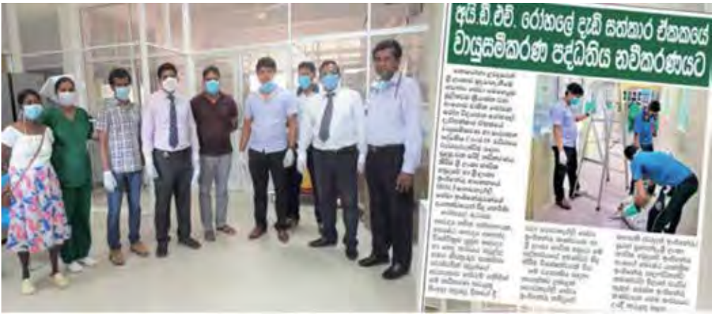
Renovation of the MVAC system in IDH Intensive Care Unit (ICU) by BSESC Engineers
